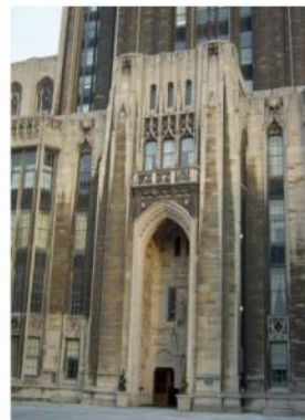
A photo of the south elevation shows the evidence of atmospheric pollution (May 2005).
