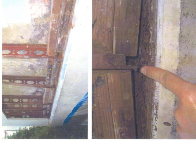
rusty sill plate
